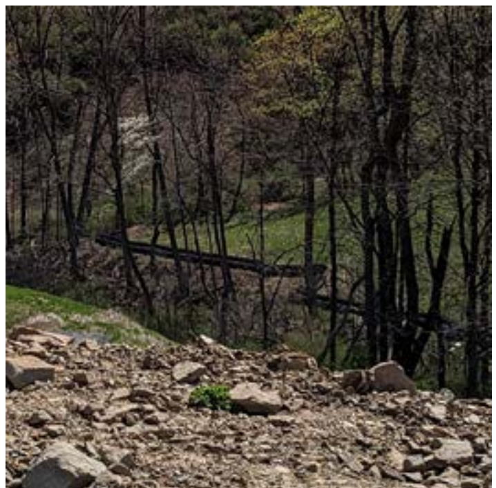
Temporary erosion controls in place near a construction site in Ohio Township. NPDES and municipal SALDOs require erosion control during construction to help mitigate the increased amount of soil entering the stormwater runoff as the ground is disturbed for construction.
