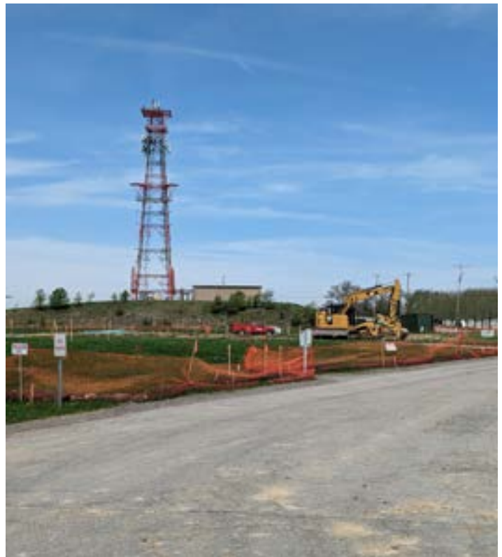
Ohio Township Public Works Crews Working on the New Park Improvements; Cell Tower in Background
