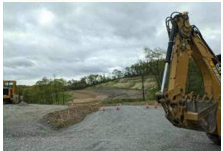
Construction at the Deerfield Estates Residential Development along Nicholson Rd in Franklin Park
