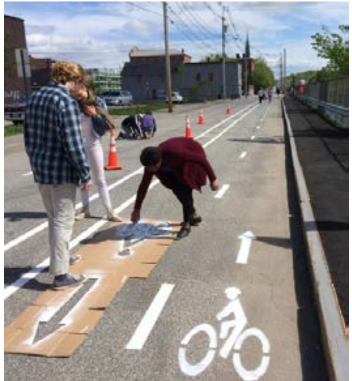
Tactical Urbanist Demonstration Project: Bates College Students Installing a Temporary Bi-Directional Bikelane in Lewiston, ME Source: Street Plans
